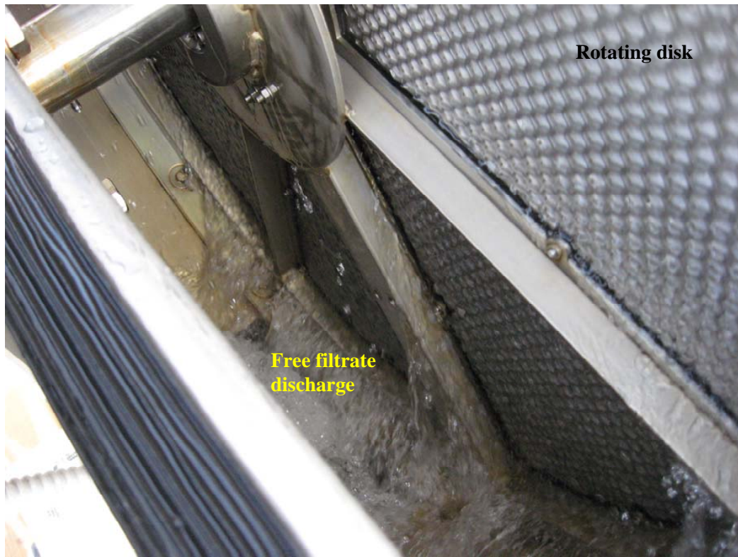
Figure 2. Free filtrate discharge on the Ultrascreen®.
